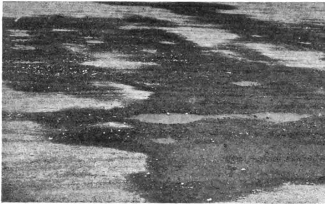
Water Shows Up Road Damage in Its True Light.
